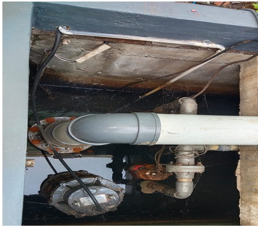
3. Panel Variable Frequency Drive (VFD)
