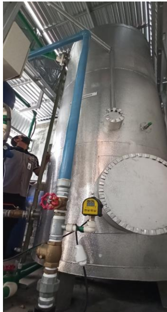
Gambar 4.7 Tangki Air Reject
