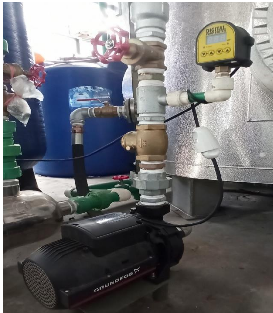
Gambar 4.9 Instalasi Pendistribusian 'Air Reject '
